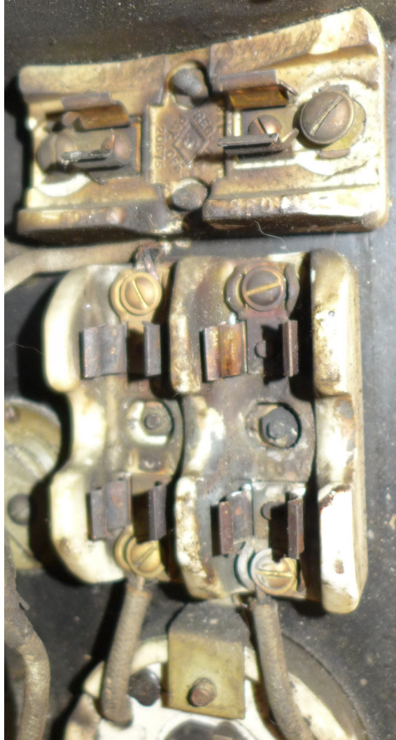
The two Fuse Holders as installed on the inside of the Right Side of the Main Electrical Enclosure
